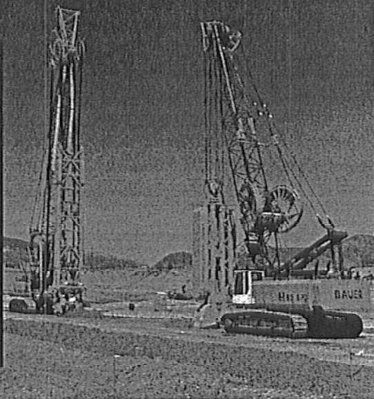
A custom-designed Bauer trench cutter and hydraulic grab at work on the Eastside Reservoir project in Southern California. Three 40m-deep plastic concrete cut-off walls were constructed to seal alluvial channels beneath the earthcore rockfill dam.
